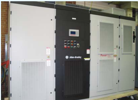
2500 hp SGBT ID Fan drive, 5kV
