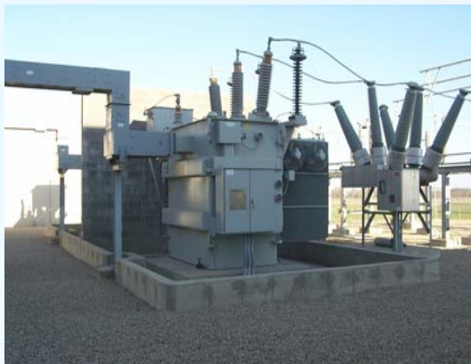
15MVA -138kV/5kV substation
