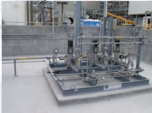
Ammonia pump skids
