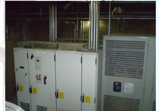
2x300hp fully redundant kiln drive VFD, 480V
