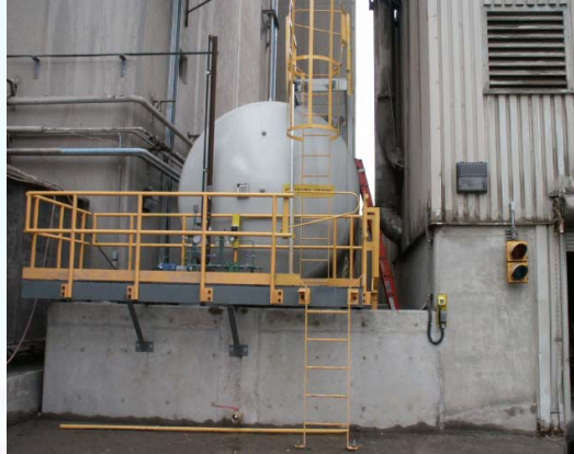
Ammonia storage tank farm 40,000lt
