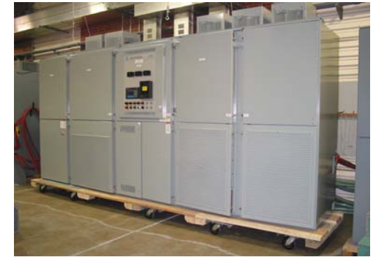
3750kW, 5 kV variable frequency drive
