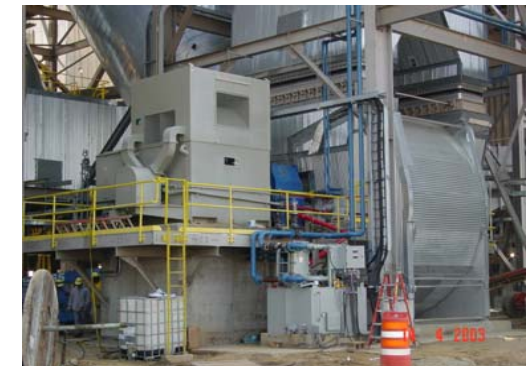
8300hp, 13.8kV, synch Motor-Fluid coupling
