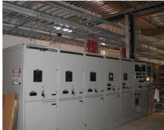
15kV Vacuum metal clad switchgear
