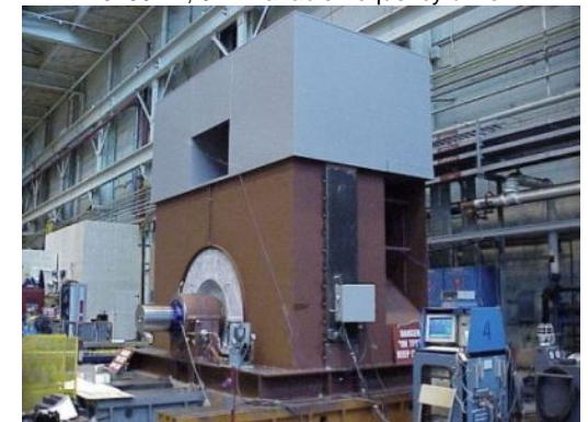
3000kW, 180 rpm, 4.16kV, ball mill synch motor
