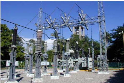
138kV, 3ph, 60 Hz incoming substation
