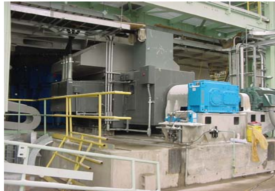
4900kW, 4.16 kV, SR ring motor drive for VRM
