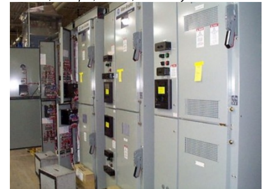
5kV VFD incoming and bypass switchgear
